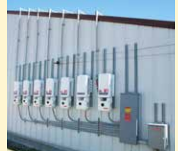
▲ A set of string inverters
