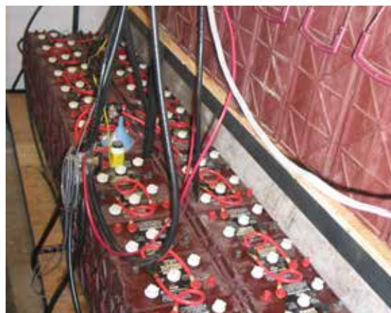
▲ A battery bank
